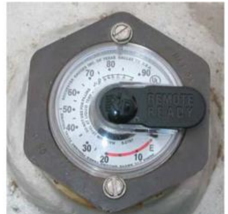
Type A dial installed, with peg at 5% mark
